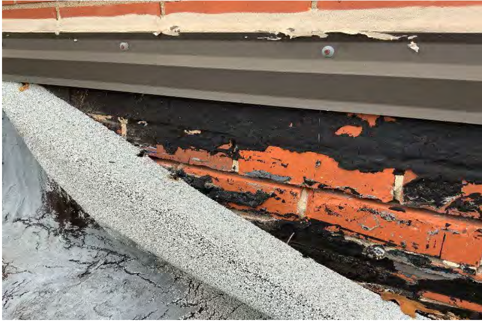
Areas below roof flashing showing signs of severe deterioration in need of tuckpointing repairs and brick replacements
