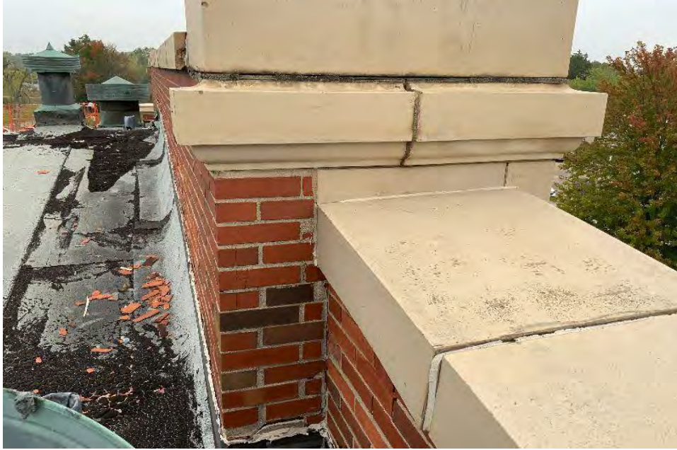
Coping joints deteriorated in need of caulk repairs
