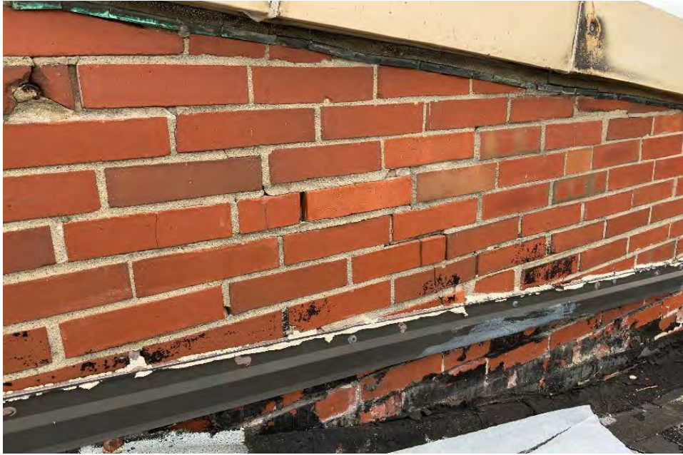
Parapet walls showing severe deterioration in need of tuckpointing repairs and brick replacements
