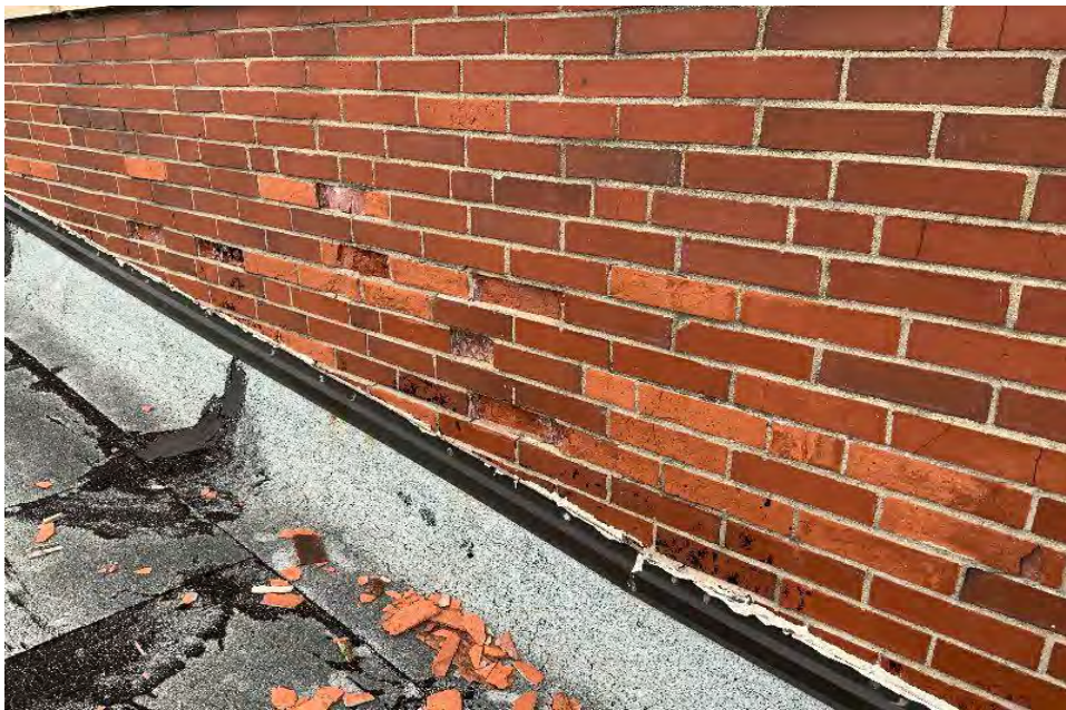
Area showing mortar deterioration in need of tuckpointing repairs
