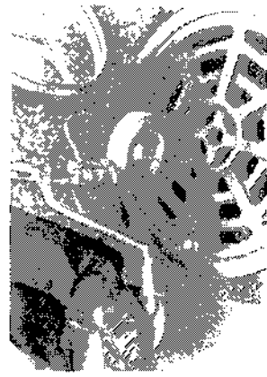
Heavily patterned manhole covers will deflect the caster wheel of wheelchairs.
