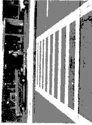
The traffic island is inaccessible to those in wheelchairs and to some of those with gait problems.
