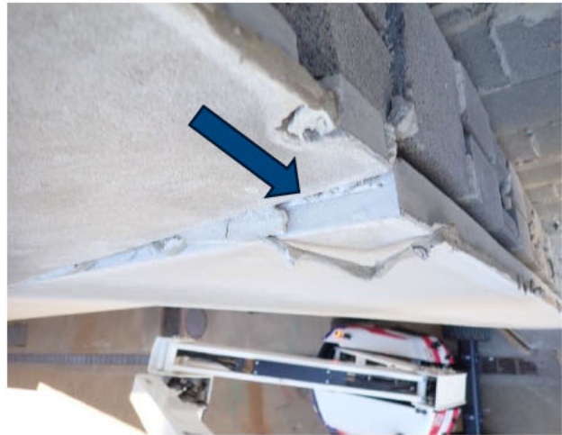
Figure 6. Impacted and rotated stone panel.
