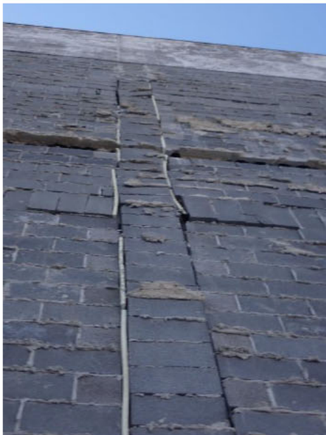
Figure 3. Misaligned and unsupported stack bonded CMU.
