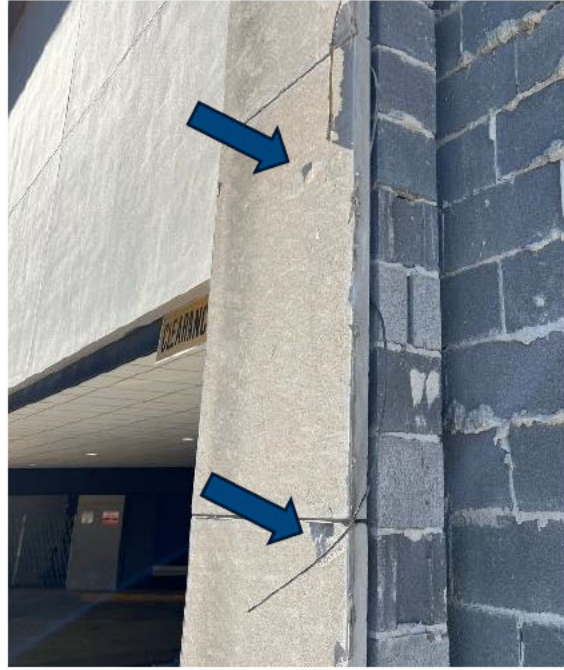
Figure 8. Locally damaged limestone panels.
