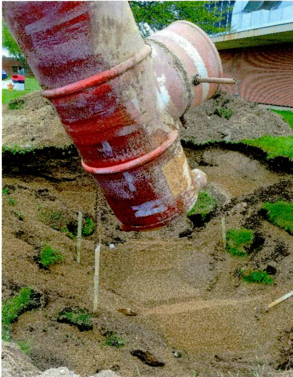
Photograph 8: View facing southeast of the removal of the UST from the excavation (May 17, 2019). Note the hold-down straps are attached to a concrete pad that was left in-place.
