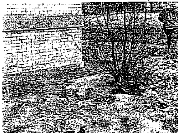
Photo #17 Typical view of the former location of a PCB-containing transformer southeast of Woods Cottage (#61) at the site.
