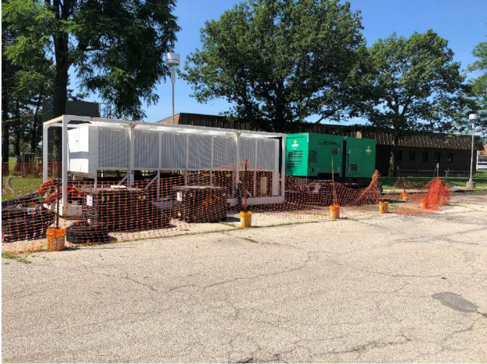
Photo 13: Portable Generators on site
