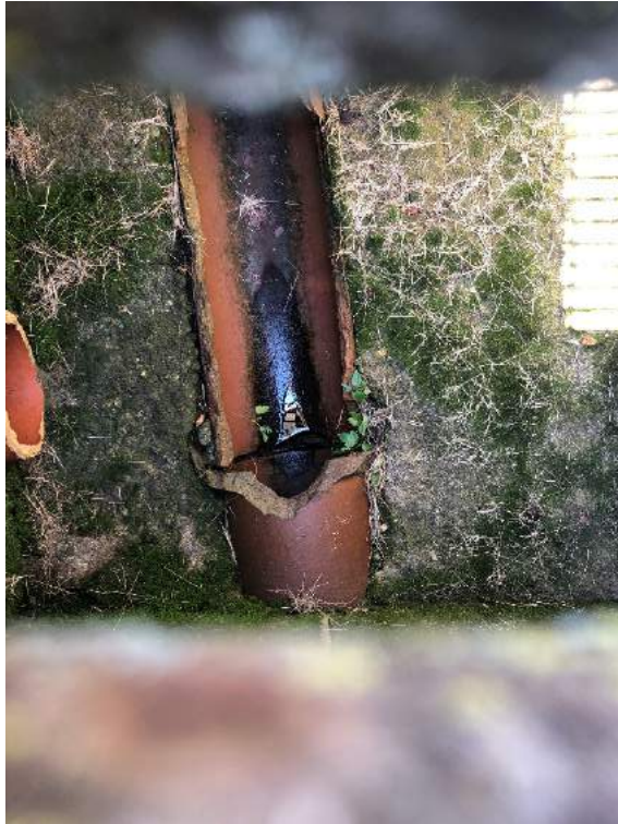
Photo 11: View of piping within the identified drain
