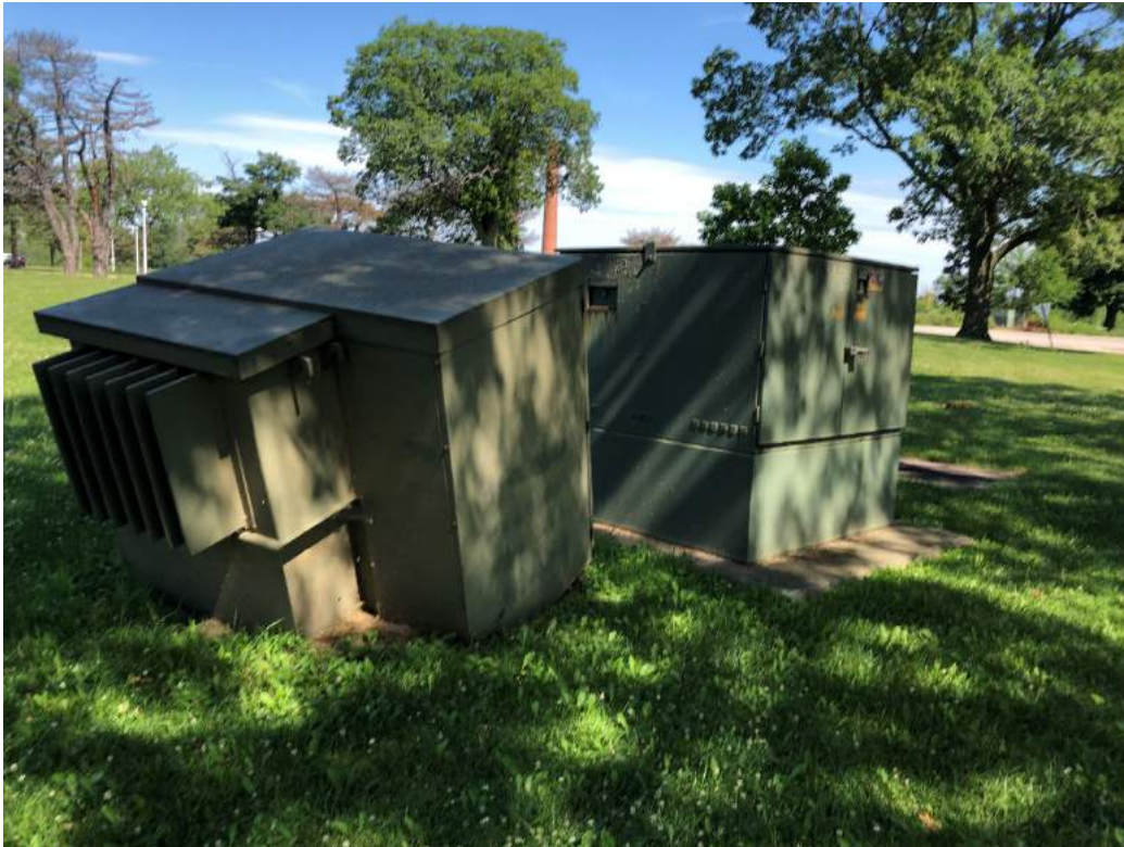
Photo 2: Transformers located in central portion of the assessment area
