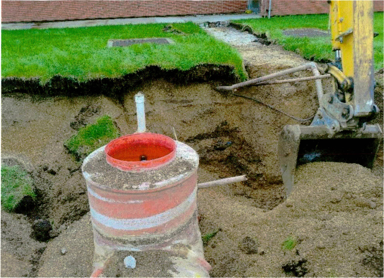
Photograph 6: View facing south showing the uncovering and removal of the product and vent lines (May 17, 2019). Note the basement vents (grates in background).
