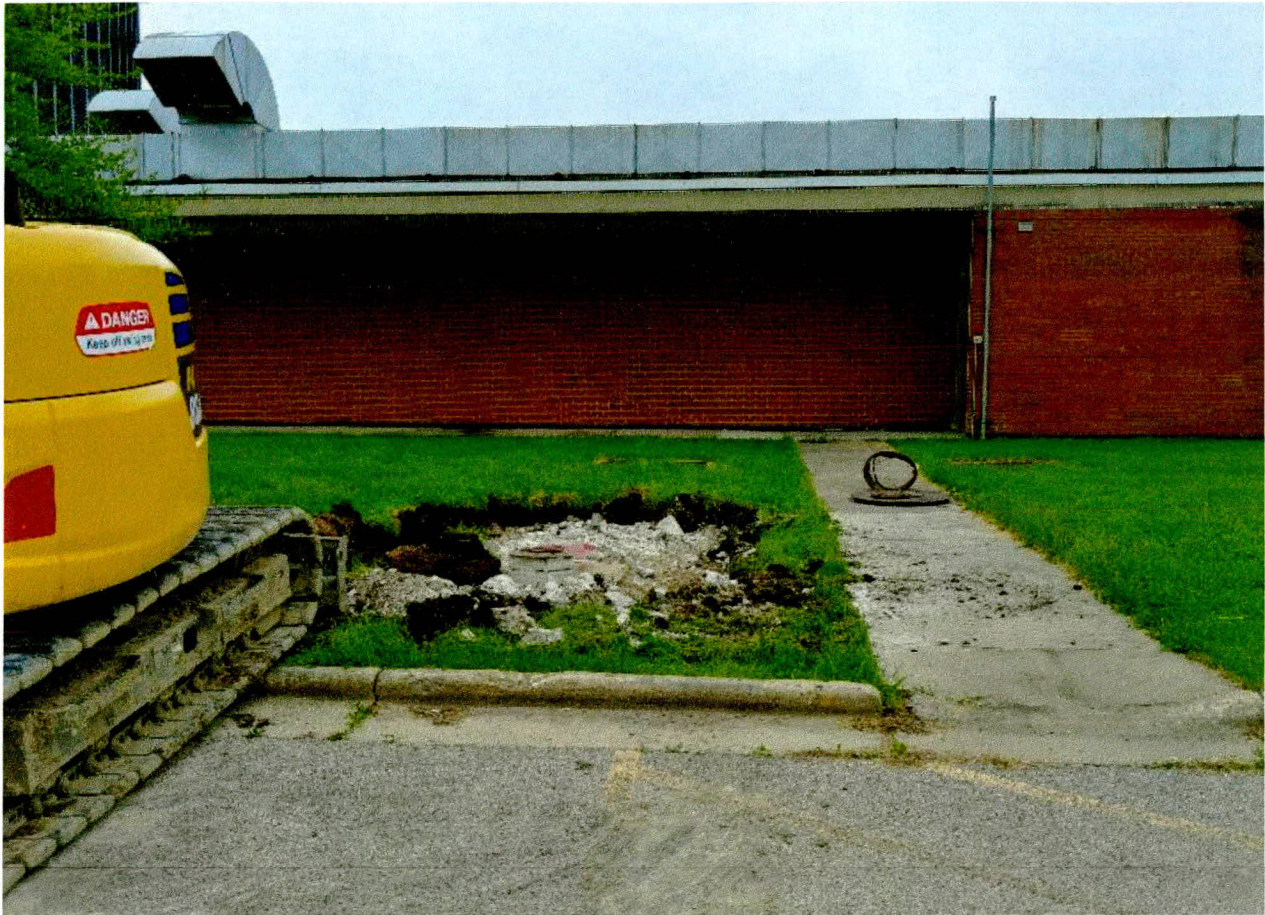
Photograph 2: View facing south showing the UST area (May 17, 2019). Note the vent line on the building.
