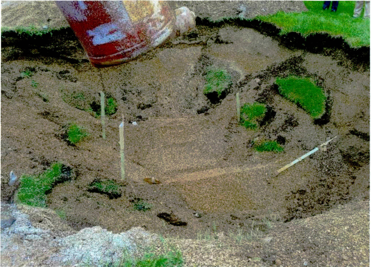
Photograph 9: View facing southeast of the removal of the UST from the excavation (May 17, 2019).
