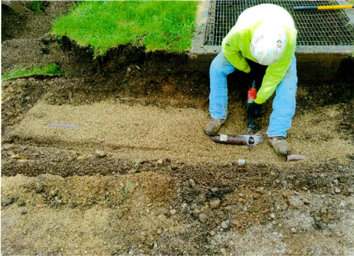
Photograph 11: View showing the removal of product line to the south of the excavation (May 17, 2019).
