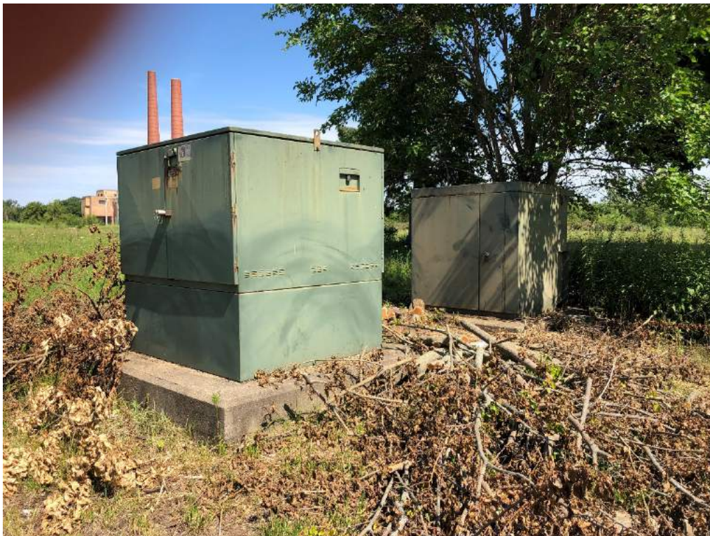
Photo 4: Transformers north of the assessment area
