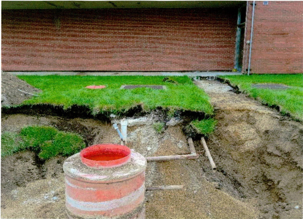
Photograph 4: View facing south showing the now uncovered tank, product line, and vent line (May 17, 2019).
