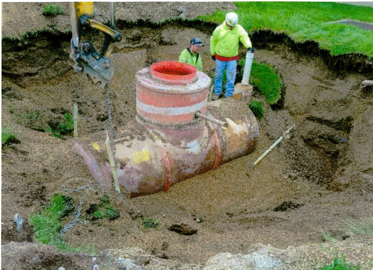
Photograph 7: View facing southwest (May 17, 2019). Attaching chain to the 1,000-gallon diesel underground storage tank for removal.
