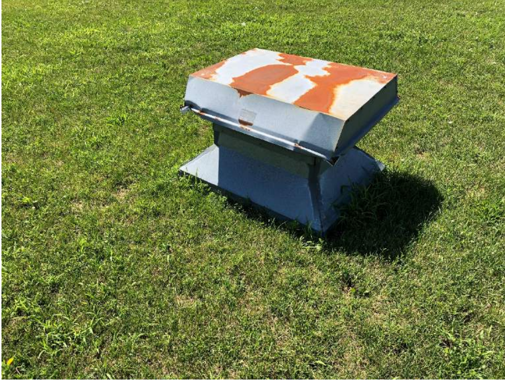
Photo 7: Steam tunnel vent western portion of assessment area
