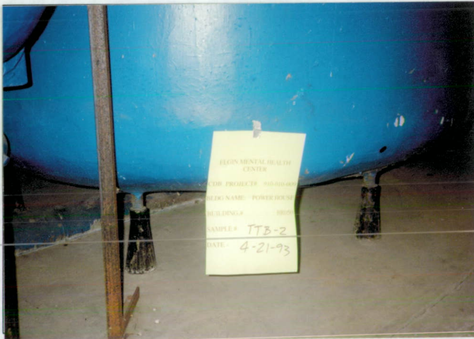
BR050-TTB-2 MAGNESIUM INSULATION ON HOLDING TANK
