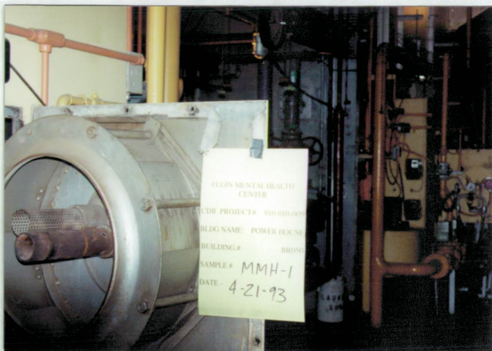
BR050-MMH-1 BOILER GASKETS
