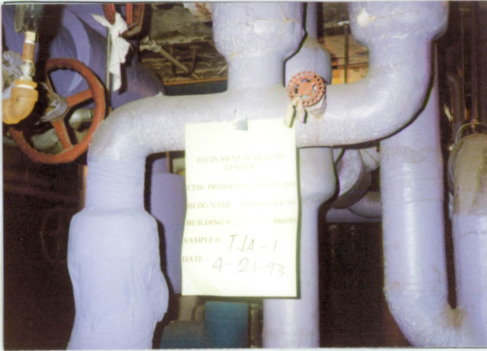
BR050-TJA-1 CEMENTITIOUS JOINT INSULATION ON MAGNESIUM PIPES
