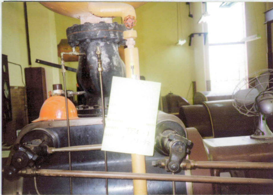
BR050-TPA-1 MAGNESIUM PIPE INSULATION
