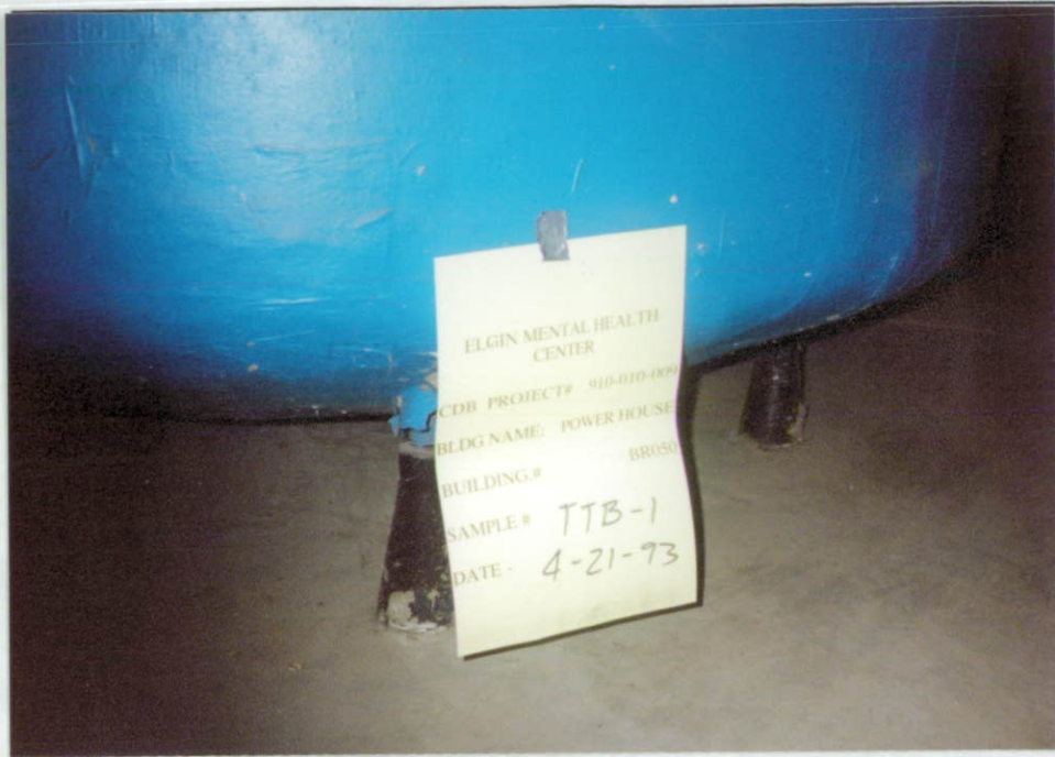
BR050-TTB-1 MAGNESIUM INSULATION ON HOLDING TANK
