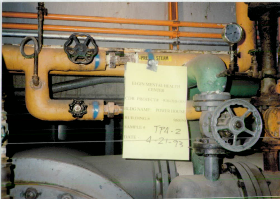
BR050-TPA-2 MAGNESIUM PIPE INSULATION
