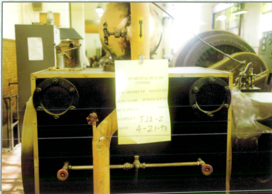
BR050-TJA-2 CEMENTITIOUS JOINT INSULATION ON MAGNESIUM PIPES
