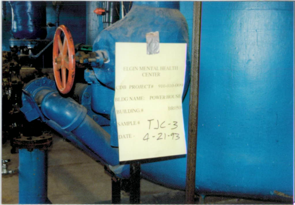
BR050-TJC-3 CEMENTITIOUS JOINT INSULATION ON AIRCELL PIPES
