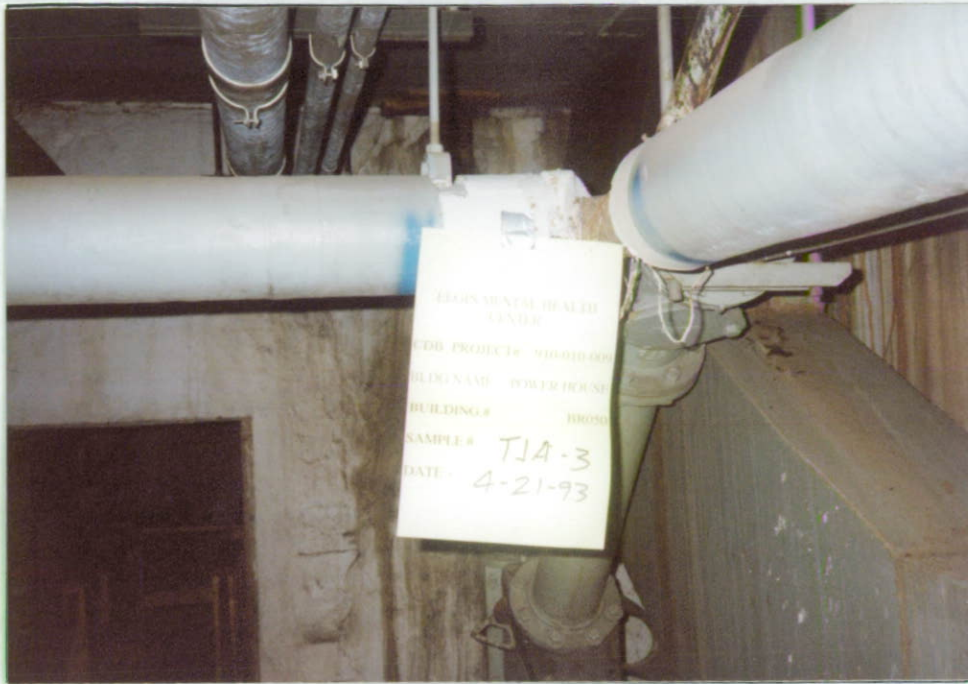
BR050-TJA-3 CEMENTITIOUS JOINT INSULATION ON MAGNESIUM PIPES
