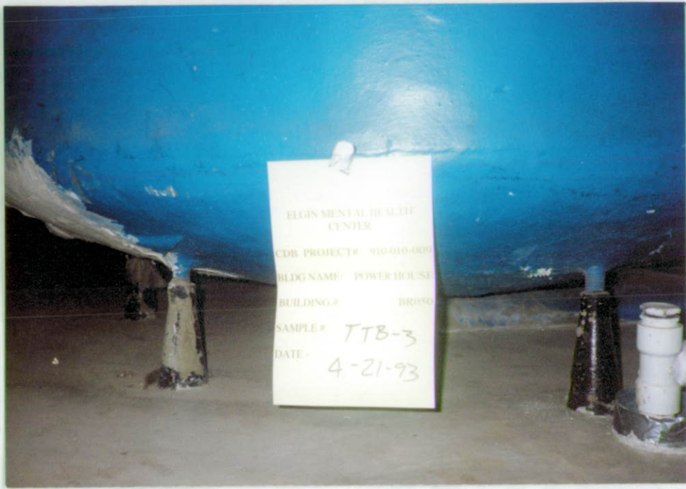
BR050-TTB-3 MAGNESIUM INSULATION ON HOLDING TANK
