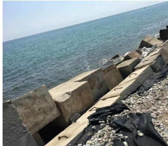
Figure 6: Failing concrete blocks shoreline protection
