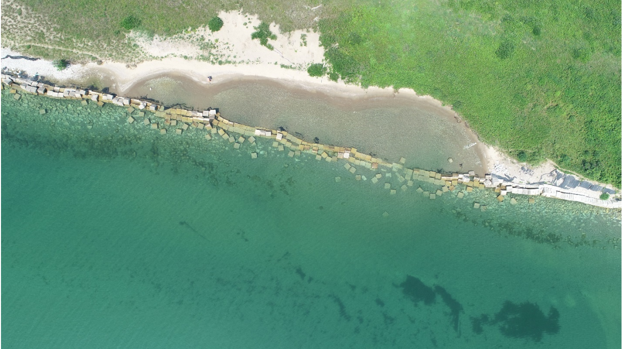
Figure F-7: Dilapidated eco-blocks ST55+00 plan view.
