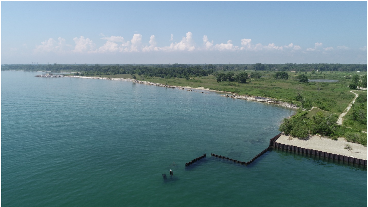
Figure F-6: Dilapidated eco-blocks ST55+00 Looking Southeast
