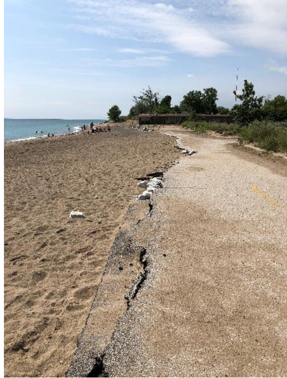
Figure E-8 Damage to Parking Lot, ST 190+50 Looking South
