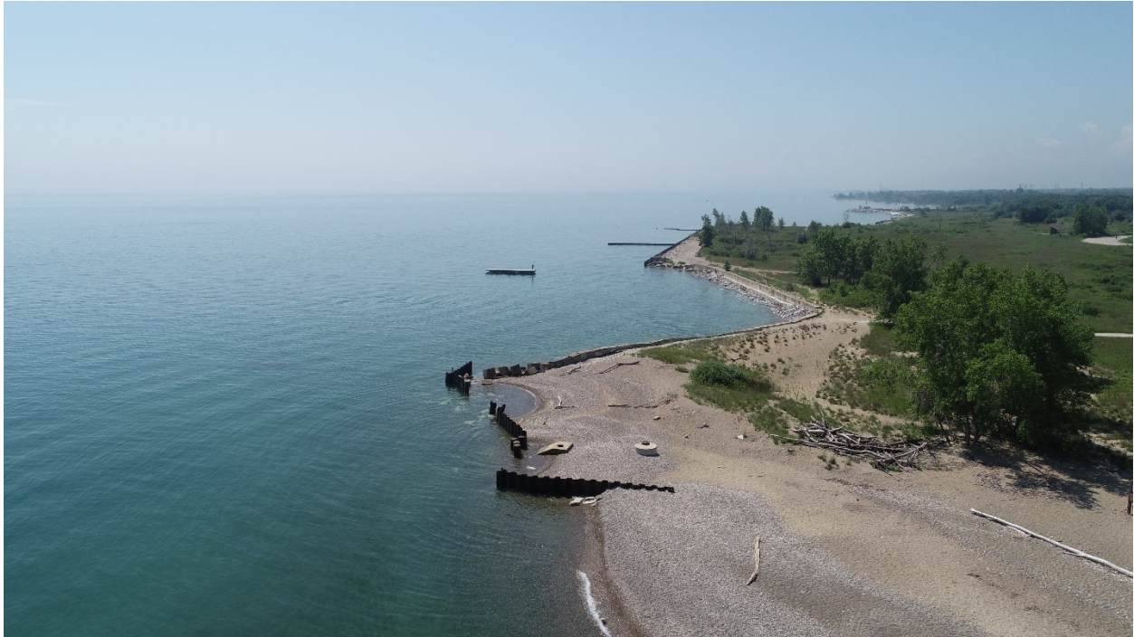
Figure F-4: Erosion behind sheetpile ST42+50 Looking Southwest.
