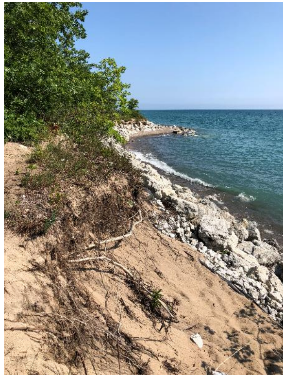
Figure E-10 Bluff Slope Failure Behind Revetment, ST 198+50
