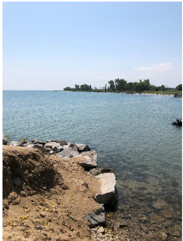
Figure E-4 Erosion at Revetment Tip, ST12+00 Looking South
