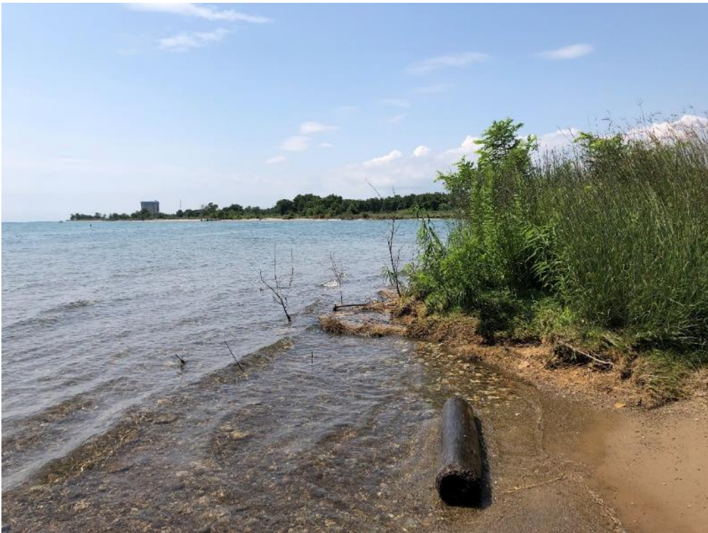
Figure E-6 Eroded Beach Behind Failed Revetment, ST71+50 Looking Southwest
