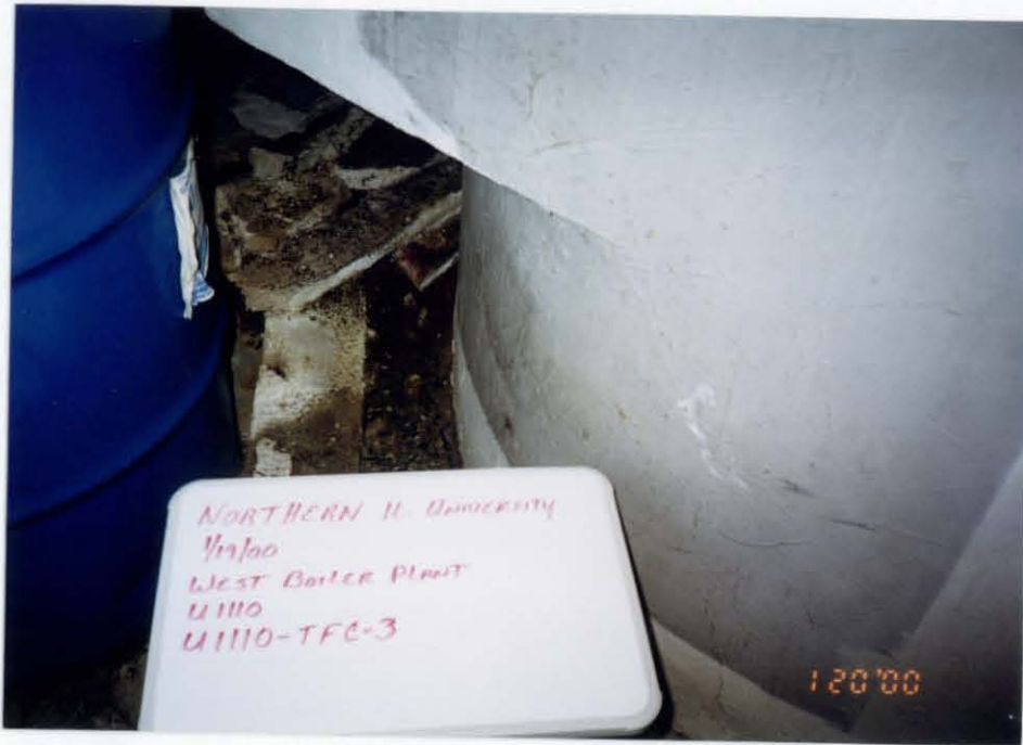
U1110 - TFB - 3 BOILER STACK INSULATION ON BOILER #3 (ADDITION #1 - 1964) (Picture is incorrect. Material designation was changed to TFB.)
