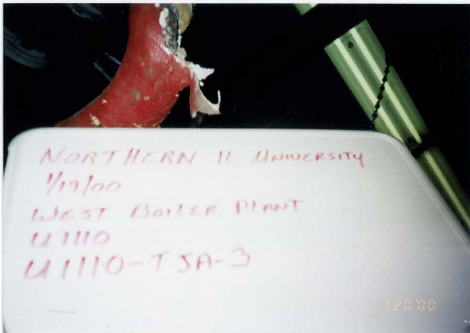
U1110 - TJA - 3 FITTINGS ON FIBERGLASS PIPE INSULATION (ORIGINAL BUILDING - 1962)
