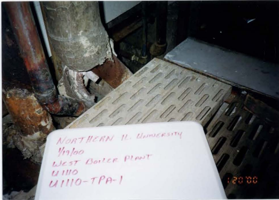
U1110 - TPA - 1 MAG-BLOCK PIPE INSULATION (ORIGINAL BUILDING - 1962)
