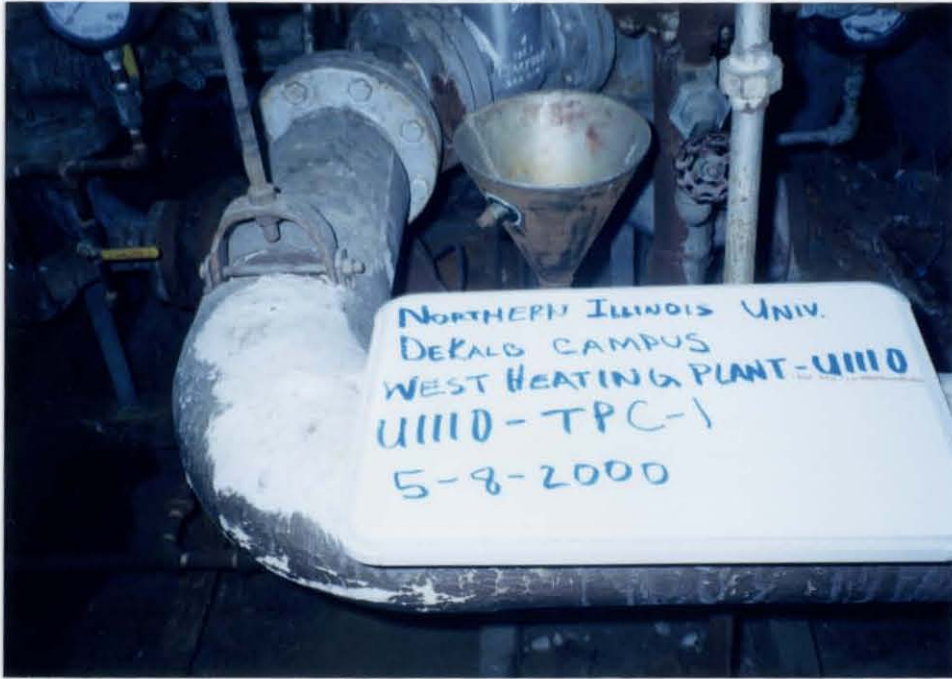
U1110 - TPC - 1 MAG-BLOCK PIPE INSULATION (ADDITION #2 - 1966)
