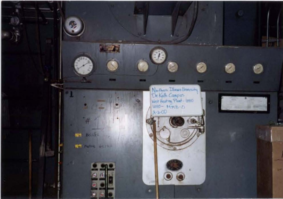
U1110 - MMB - 0 GASKETS ON BOILERS #1 AND #2 (ORIGINAL BUILDING - 1962)
