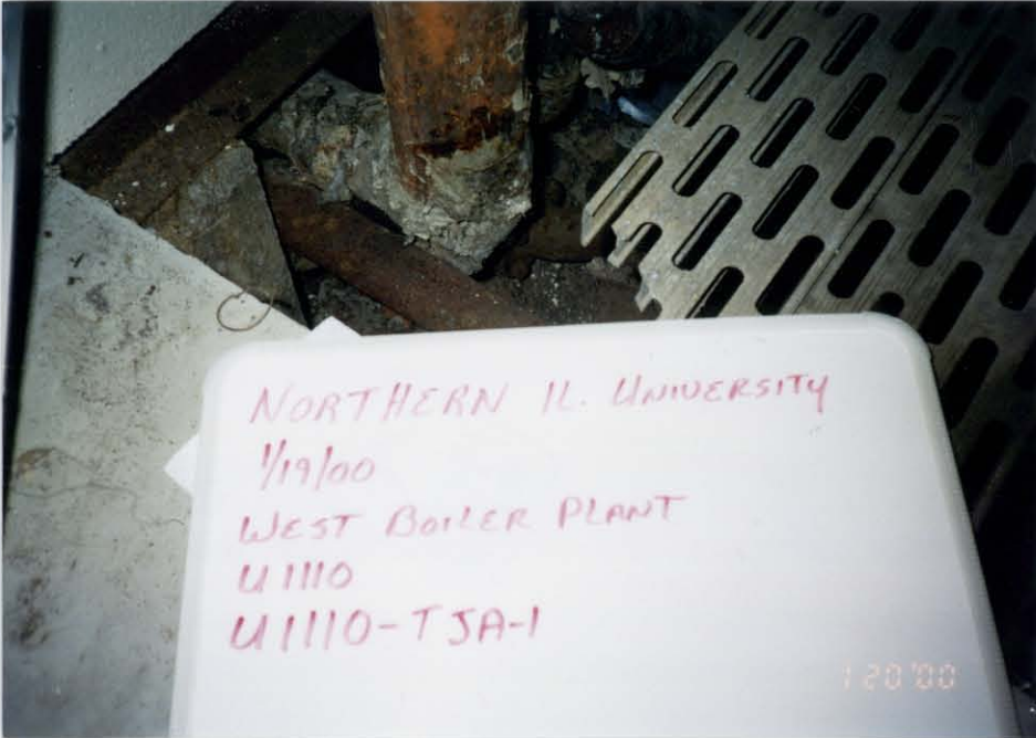
U1110 - TJA - 1 FITTINGS ON FIBERGLASS PIPE INSULATION (ORIGINAL BUILDING - 1962)
