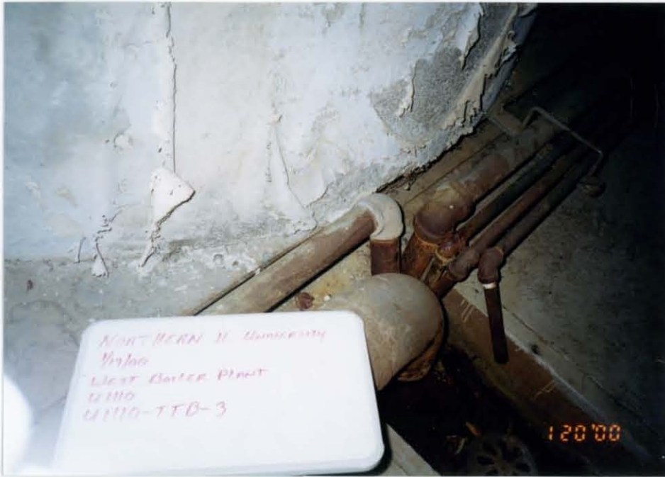
U1110 - TTB - 3 RECEIVER TANK INSULATION (ADDITION #1 - 1964)
