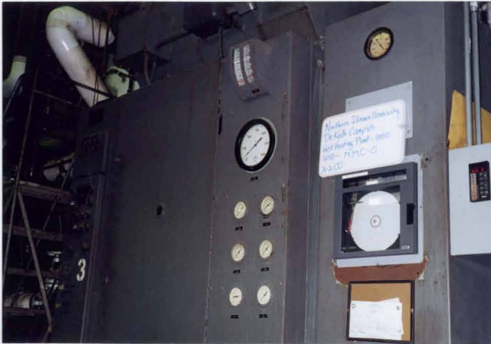
U1110 - MMC - 0 GASKETS ON BOILER #3 (ADDITION #1 - 1964)
